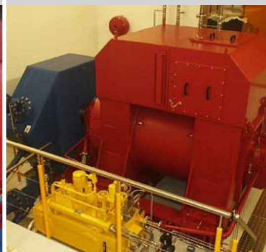
Switzerland DSG125 (2500kVA)
